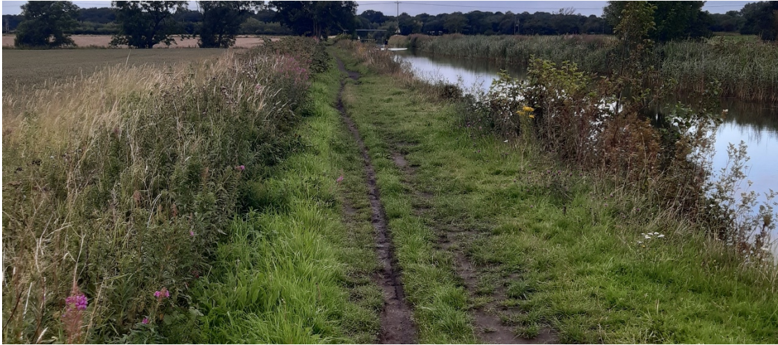
7 - Towpath condition North of Morris Lane
