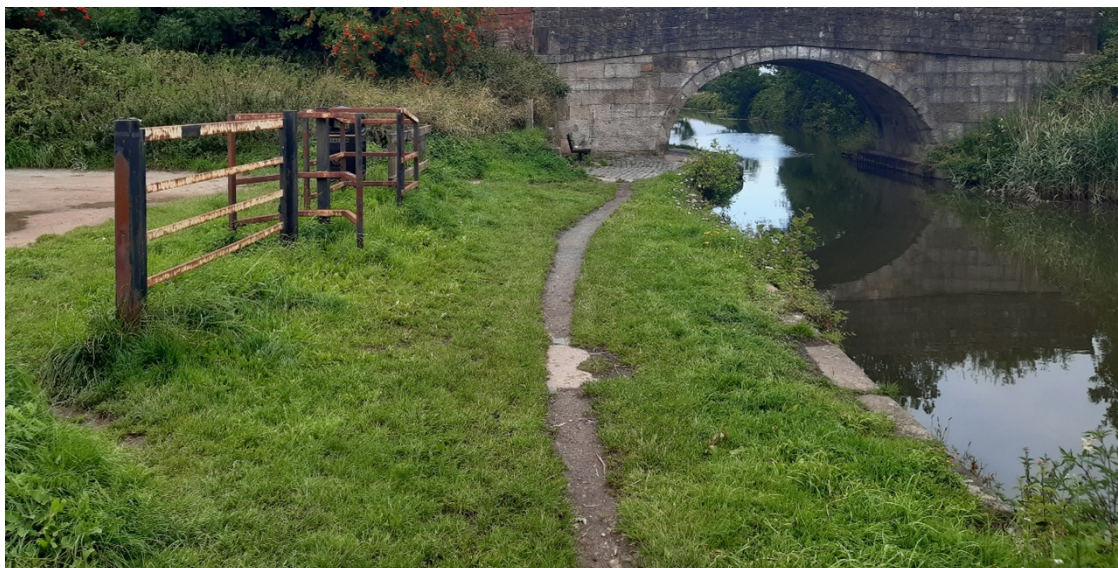
6 - Morris Lane Bridge
